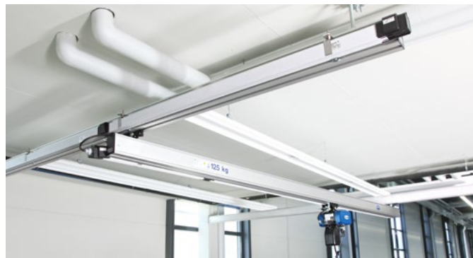
Crane system with conductor line to supply a chain hoist
