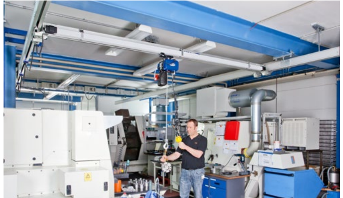
Low ceiling mounted aluminum single bridge crane system with conductor line to accommodate the low ceiling height
